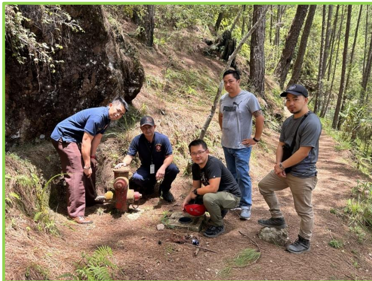
The Joint Inspection and Evaluation of Fire Hydrants and Standpipes of the JHMC and CJHDevCo at the Camp John Hay Forest.
