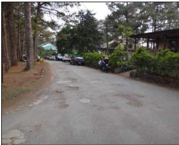
Photo of the area before the repair
