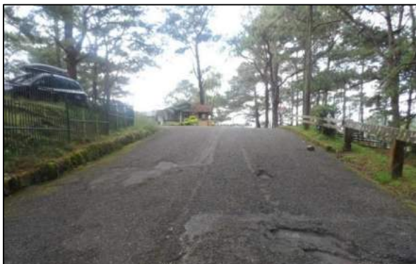
Photo of the area before the repair
